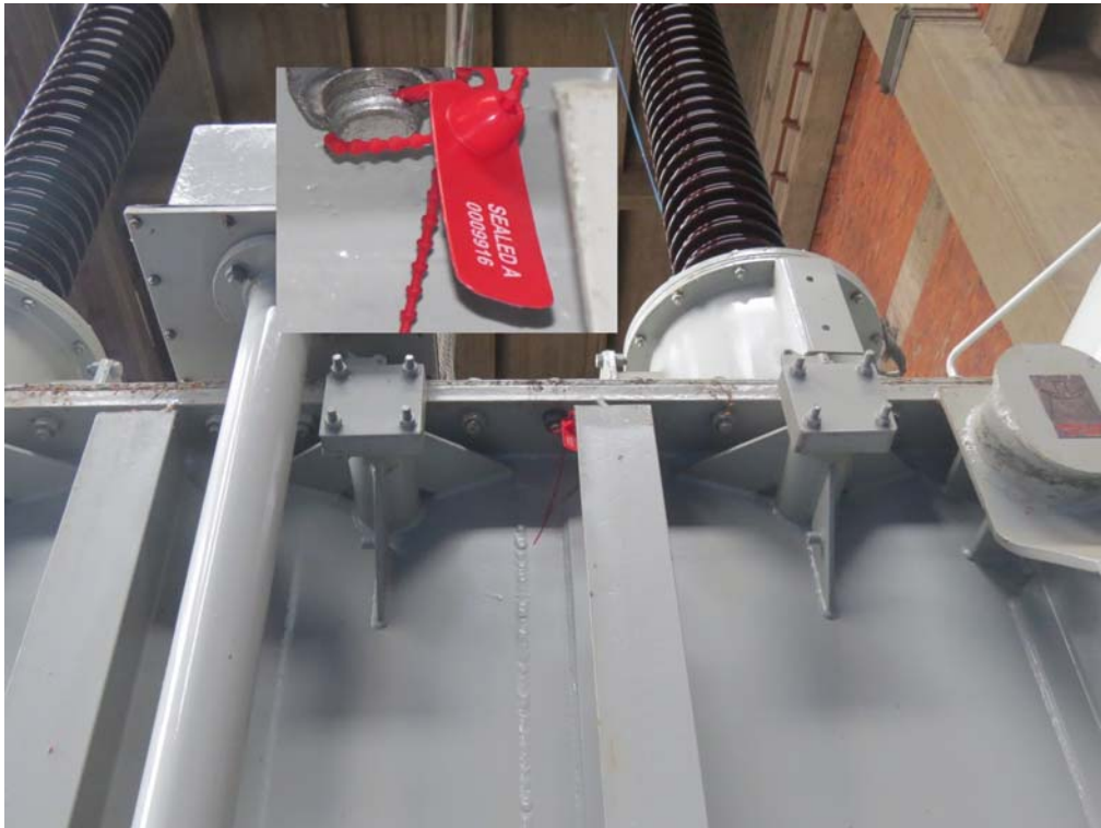
Photo No.6 Sealed 0009916 After tests
