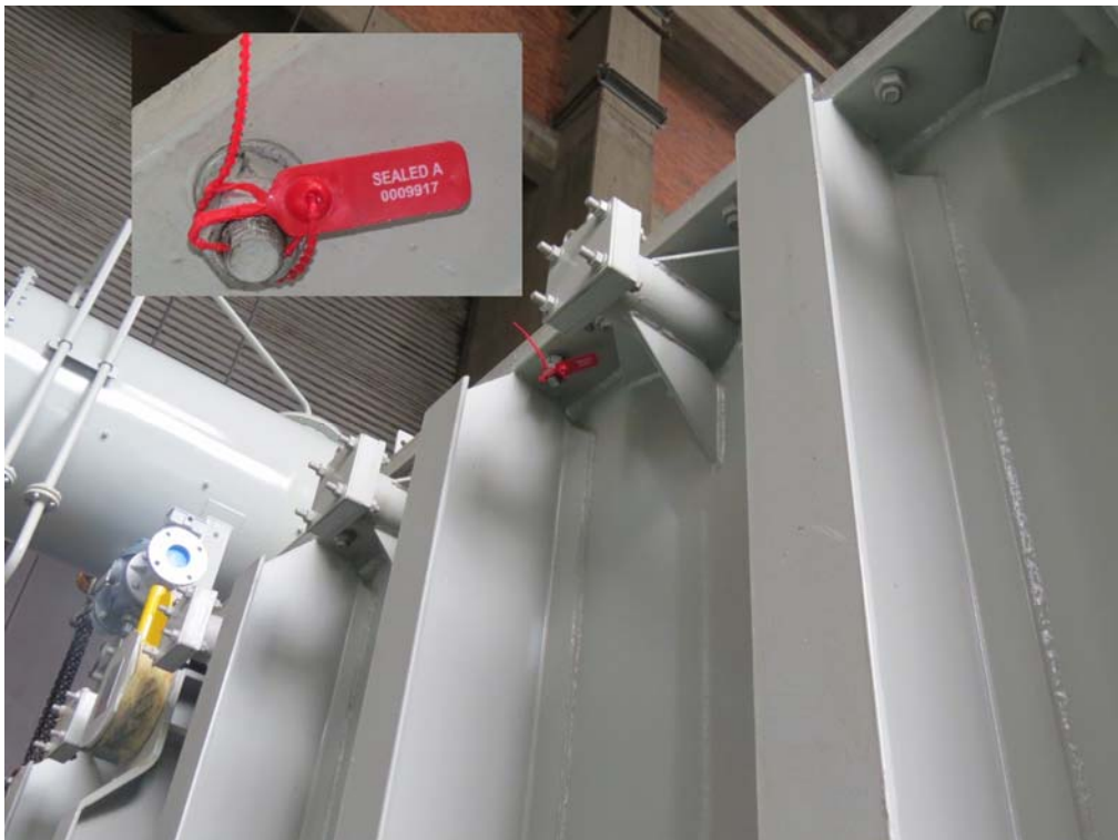
Photo No.7 Sealed 0009917 After tests
