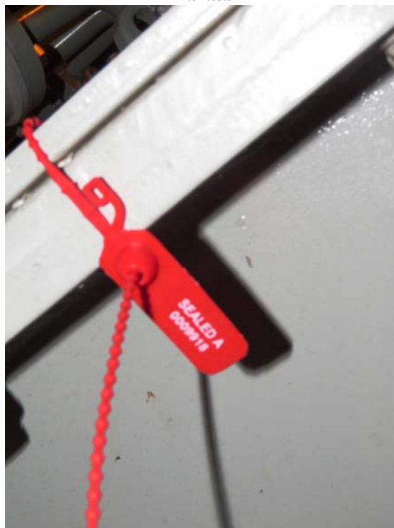
Photo no. 5 Sealed 0009918 After tests
